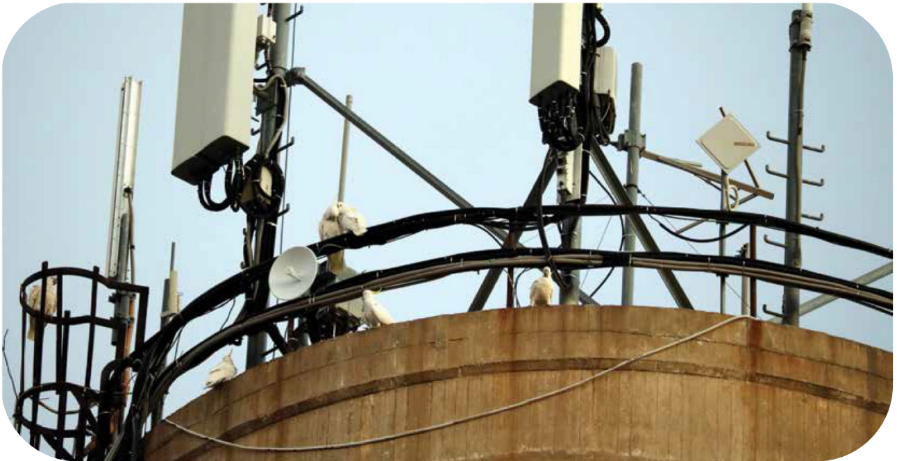
Balonne Shire mobile towers. Credit: SWQROC.
